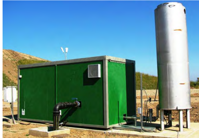
Figure 3-65: Sample landfill gas treatment facility at landfill
