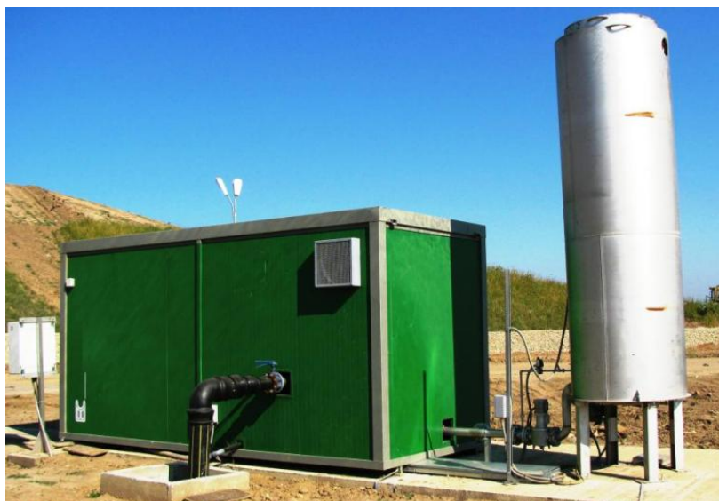
Figure 3-64: Sample landfill gas treatment facility at landfill
