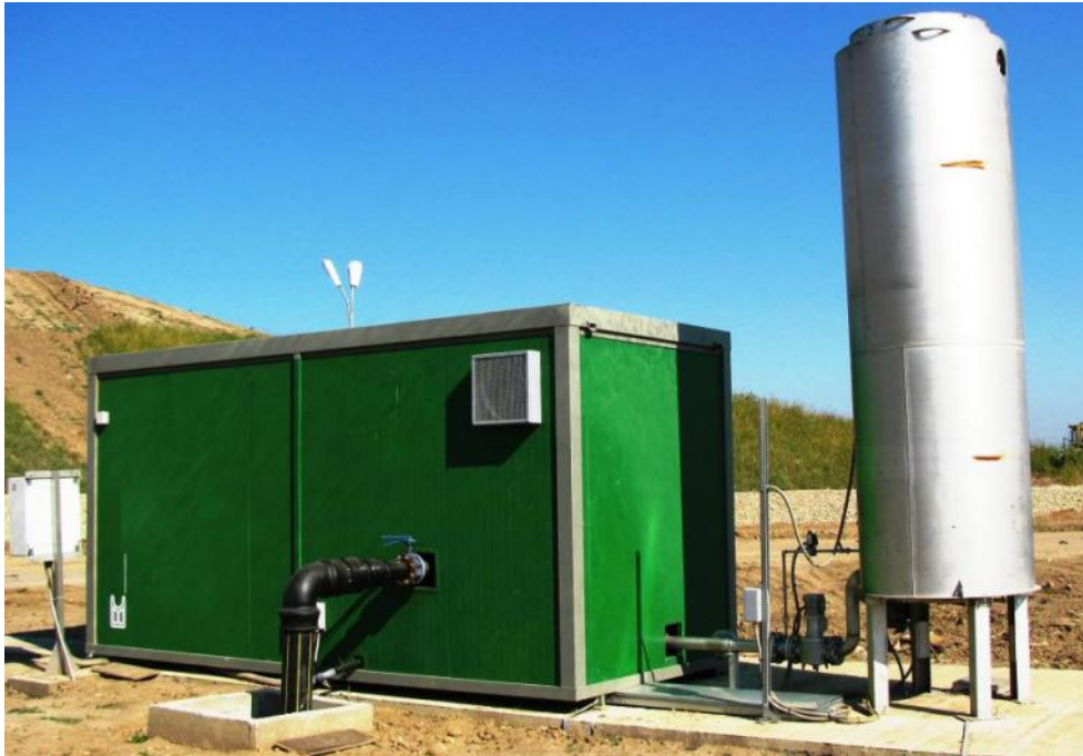
Figure 3-63: Sample landfill gas treatment facility at landfill
