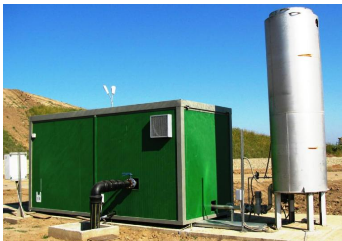
Figure 3-57: Sample landfill gas treatment facility at landfill
