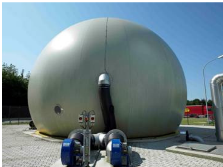
Figure 3-87: Storage tank of biogas from a waste fermentator
