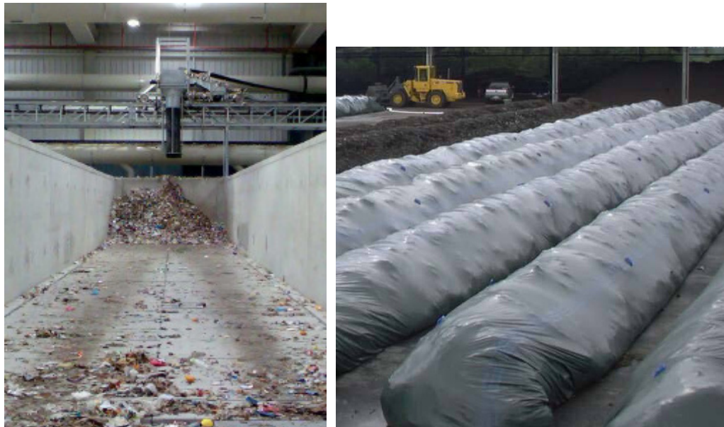
Figure 3-85: a) composting in tunnel (lanes) with perforated aeration floor, b) composting in bags
