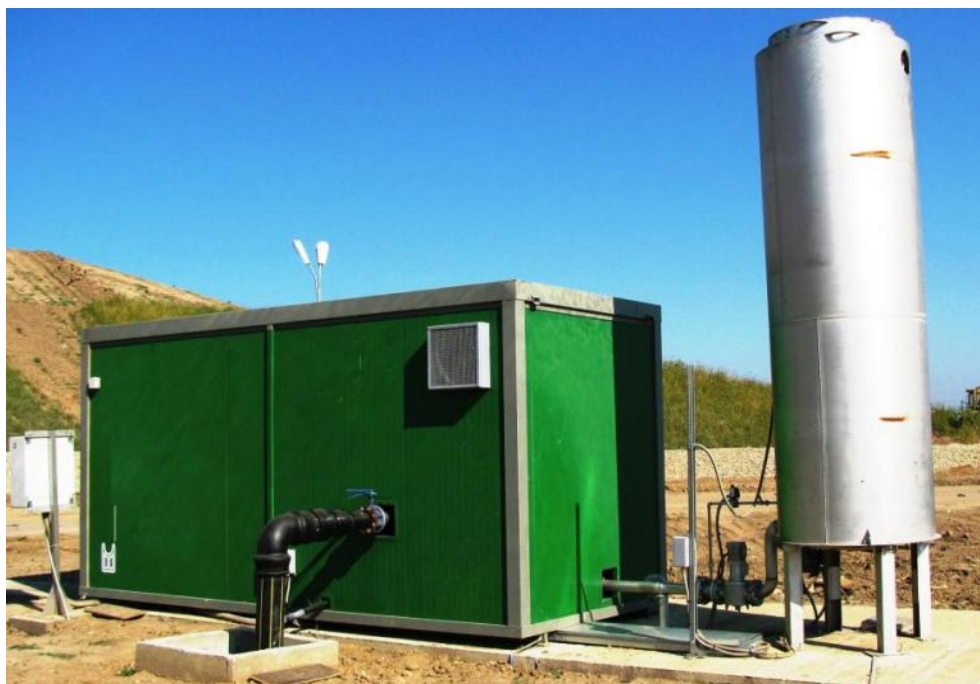
Figure 3-95: Sample landfill gas treatment facility at landfill
