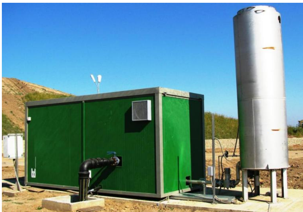
Figure 3-97: Sample landfill gas treatment facility at landfill
