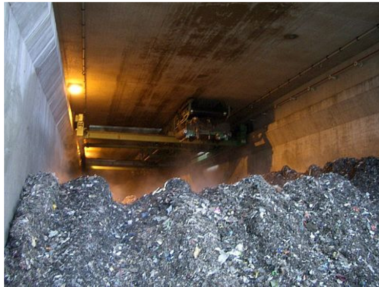
Figure 3-82: MBT composting tunnel
