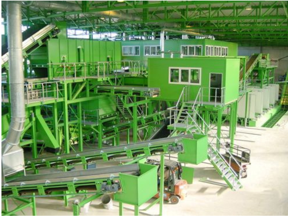
Figure 3-80: MBT plant interior
