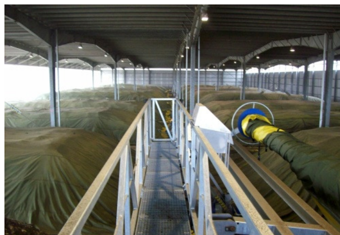
Figure 3-75: Aerated covered heaps (indoors)
