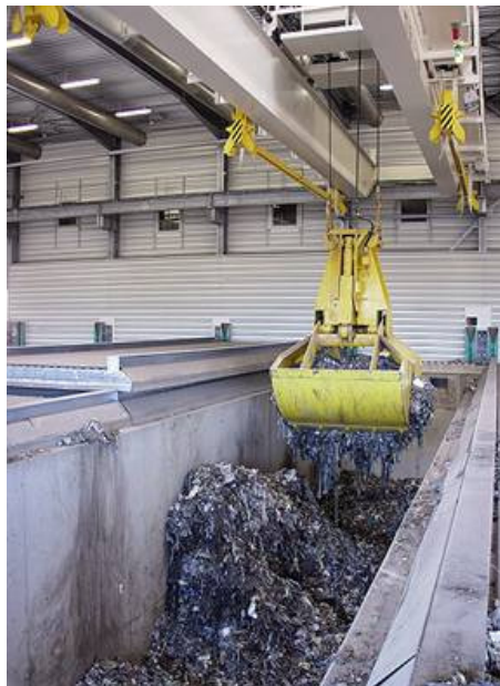
Figure 3-86: a) biodrying of mixed waste in closed boxes, b) windrow composting in building
