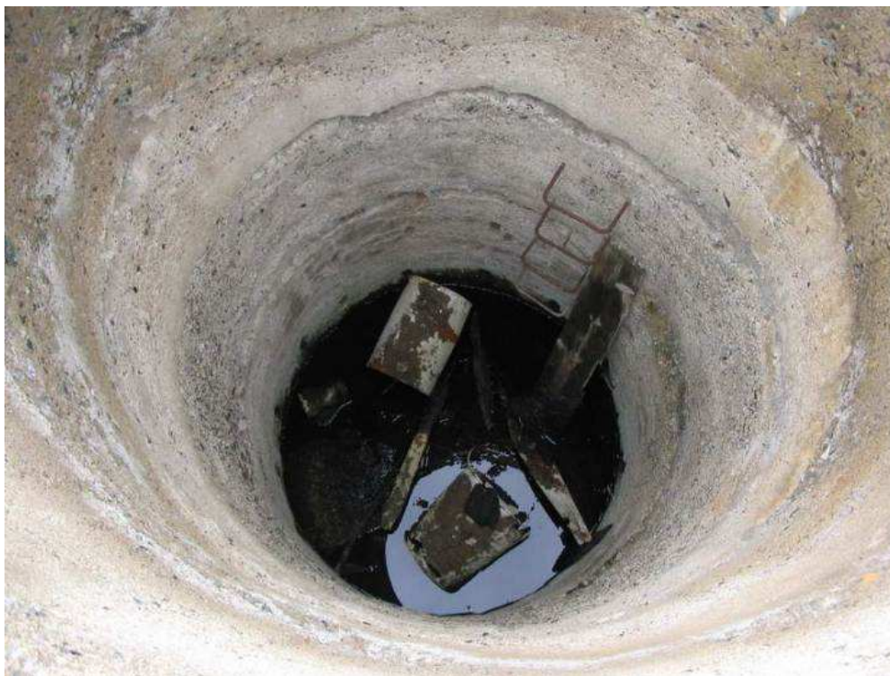
Photo 3.4 – Unprotected well at former roasting facility
