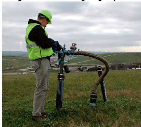
Figure 7-50: Monitoring the gas system
