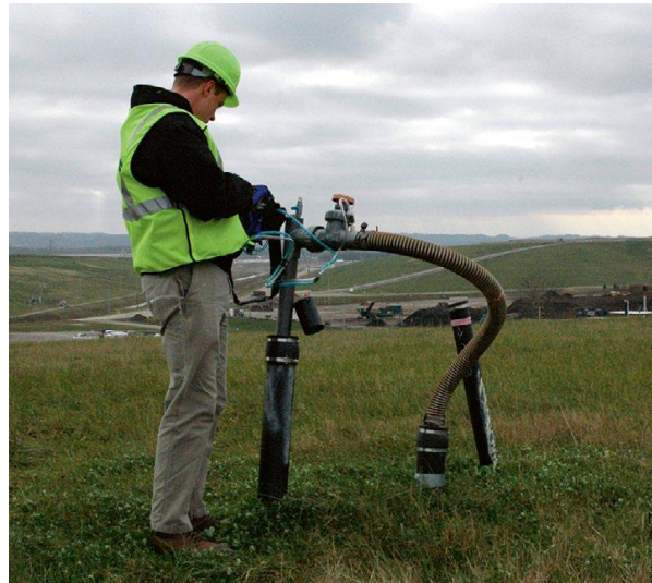
Figure 7-55: Monitoring the gas system
