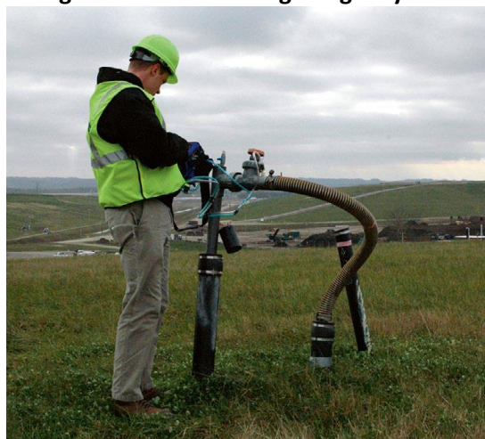
Figure 7-51:Monitoring the gas system
